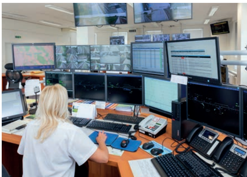
Dispatcher's workplace in Břeclav equipped with AŽD technologies.
